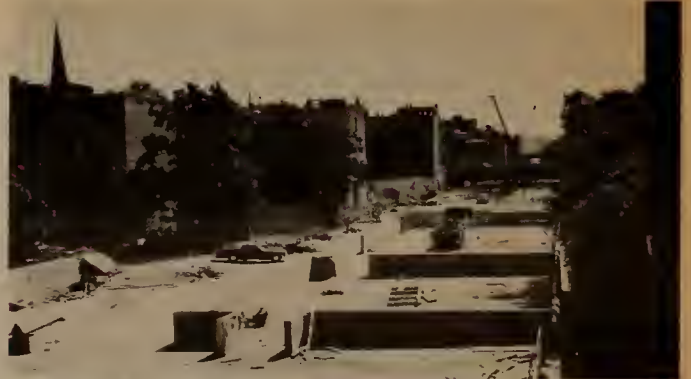
Retaining walls for the landscaping on the Cover are in place in Section I.
